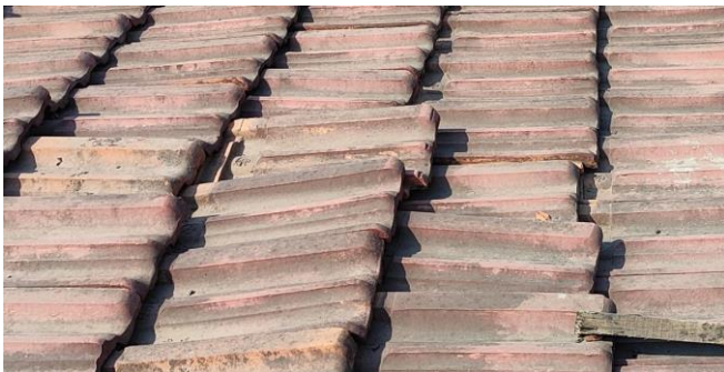
Figure 11: Misalignment of Mangalore Tile
