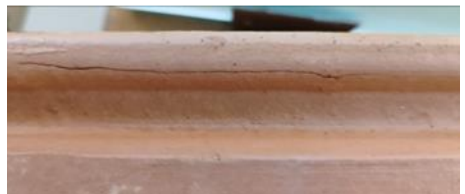
Figure 10: Distresses Present in Mangalore Tile
